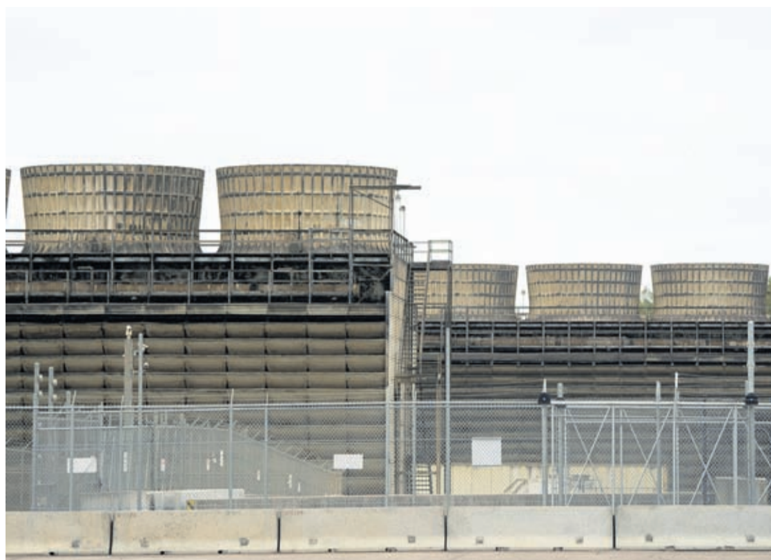
Cooling towers release heat generated by boiling water reactors at Xcel Energy's Nuclear Generating Plant on Oct. 2, 2019, in Monticello, Minn.
